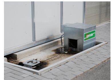
Drive unit on floor
