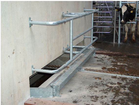
Safety gate for discharge
