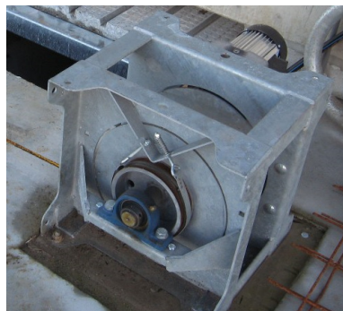
Drive unit mounted on floor
