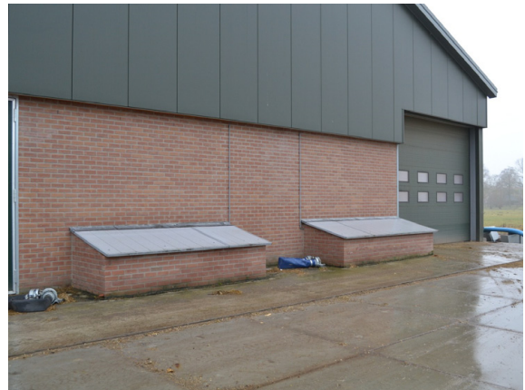
Brick container on top of discharge
